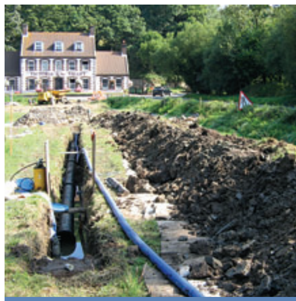
St Peter's Valley - replacement 300mm diameter raw water transfer main and new 90mm diameter treated water main
