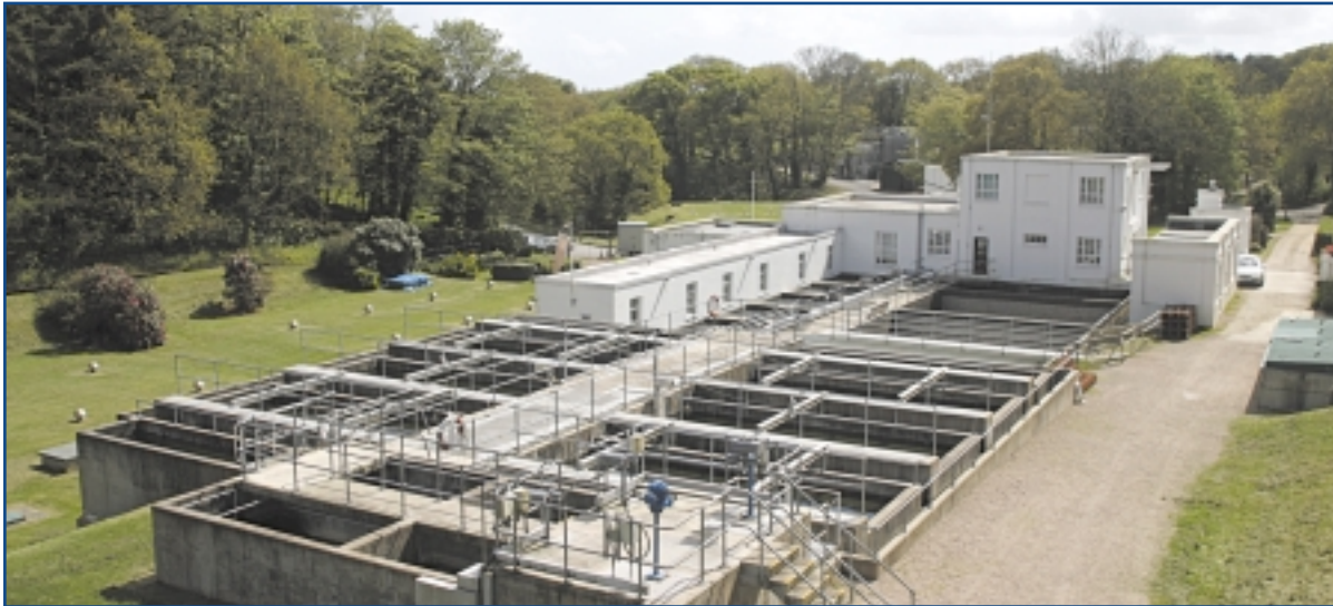
Handois Treatment Works
